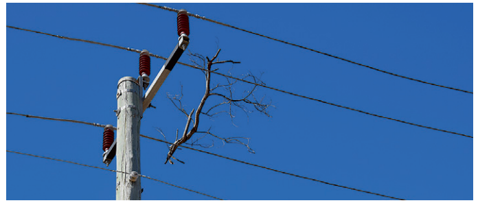
Fallen branches often cause temporary faults on powerlines
